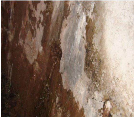
Seepage in Channel
