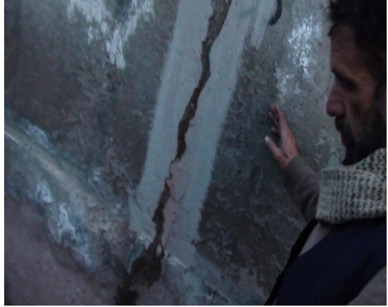
Cracks in Channel
