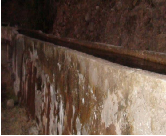
Seepage in Channel
